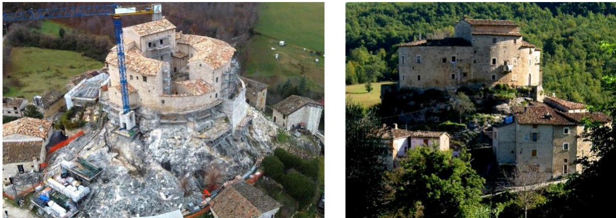
Figure 9: Castel di Luco (di Luco Castle), in Acquasanta Terme (Ascoli Piceno), ICCD code number 1100060612, date of compiling 1994, date of updating 2018: the castle under works of repair of damages and refurbishment, started after 2018 (left), and the castle today (right).
