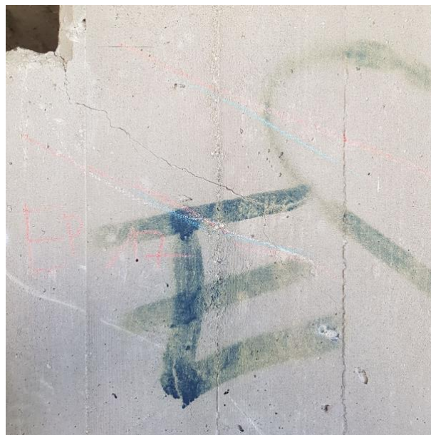
Figure 25: Crack and crack similar structures.
