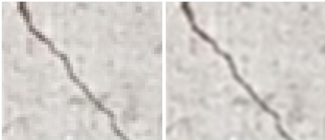
Figure 13: Crop of a crack image (original left, resampled image right).
