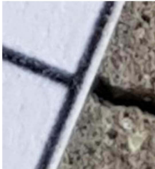
Figure 29: Detail view of crack measurement
