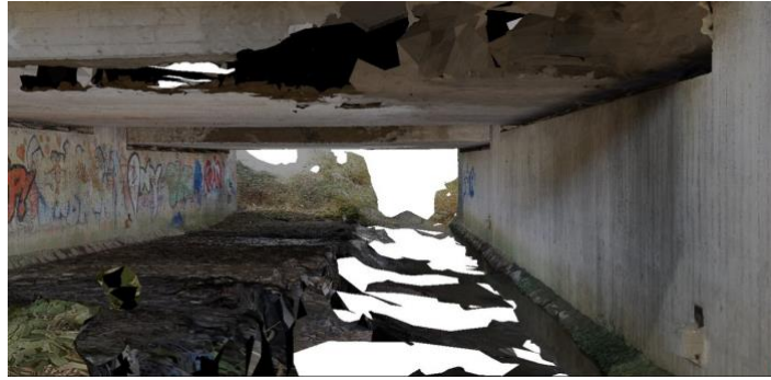
Figure 11: Perspective of the underside of the textured mesh including problems in the ceiling area.
