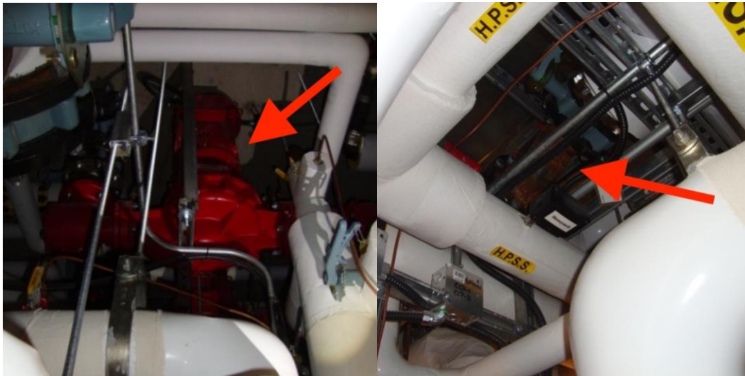
FIG. 2: Examples of maintenance access-related issues as highlighted by O&M practitioners in the CIRS building
