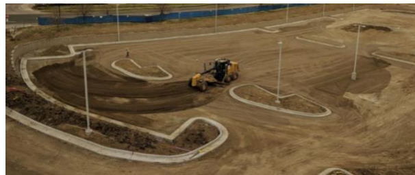
Figure 6: A grader with a Trimble GCS900 Machine Control system working on the northwest corner of the parking lot.
