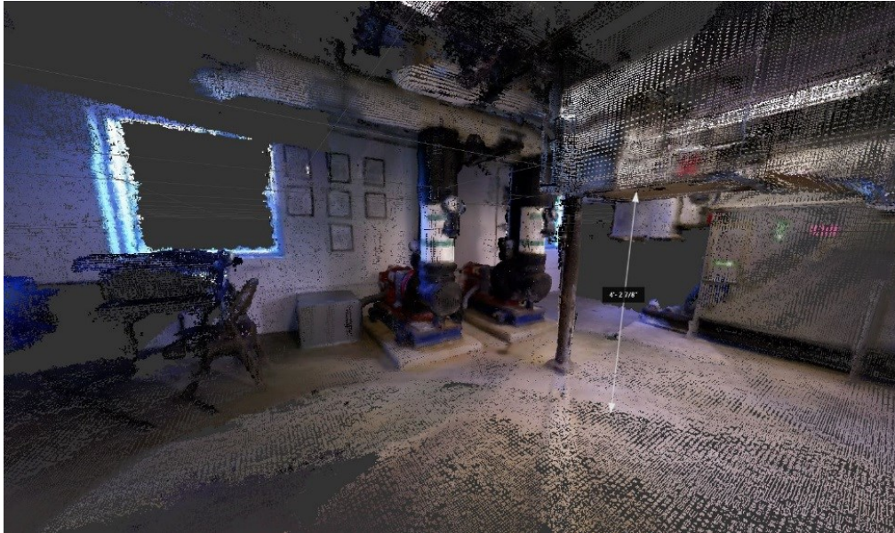
FIG. 2: Point cloud of a mechanical room captured using infrared scanning and photogrammetry techniques.
