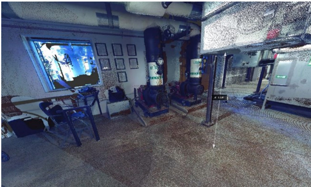
FIG. 1: Point Cloud of a mechanical room captured using a traditional phase shift laser scanner.
