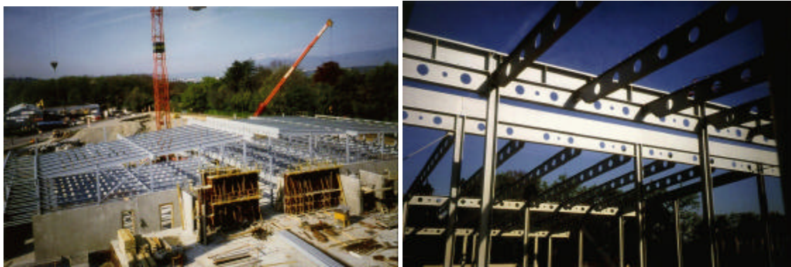
FIG. 17: Construction site of the steel-framed building example. Holes in beams hold ventilation ducts.
